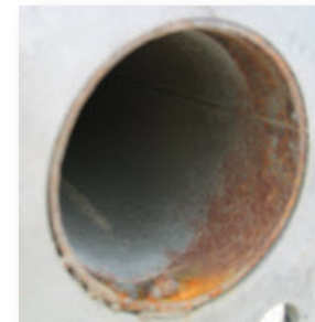
Pre-galvanized, welded steel truss frame by a competing supplier, shows inside rust.
