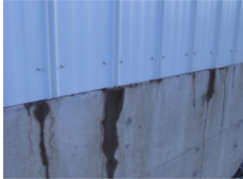
Failure of moisture/air seal in standard frame building
