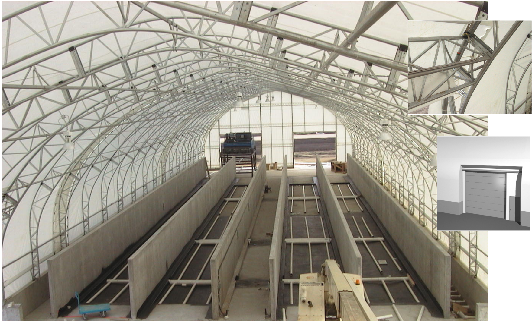
University of Alberta, Edmonton -- Farm Composting Facility Mod HP60 X 230
